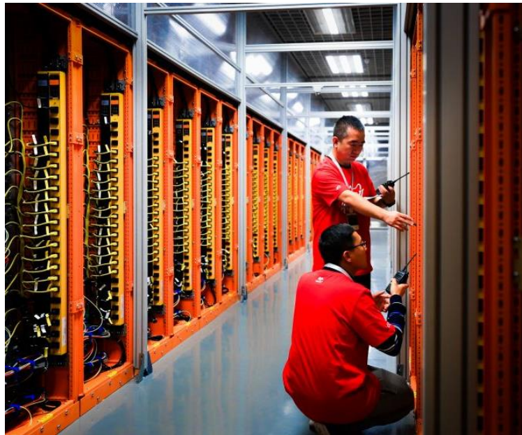
Alibaba Cloud Engineers Working In Data Centers
